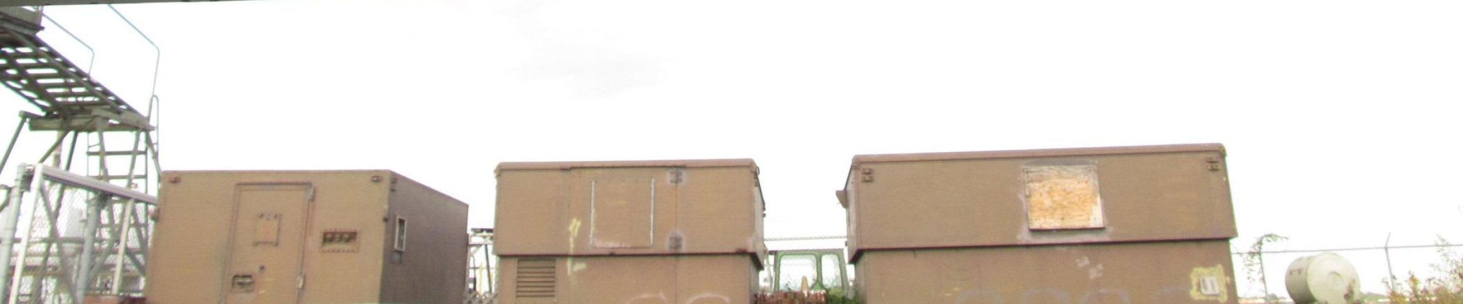
Hole In Bottom Of Left Stabilizer
